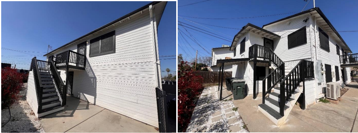
Southside & South East of the building: Staircases with premature updates, and exterior paint and trim for approval.
