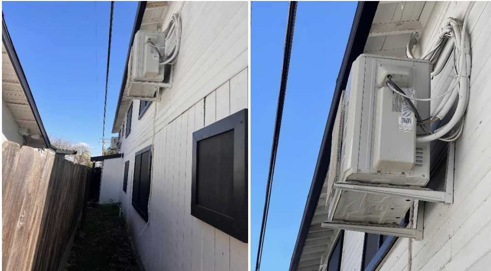
North Side of the Building: Remove/relocated HVAC (premature installation) to ground level. Will provide covering for wire, cables, lines, etc.
