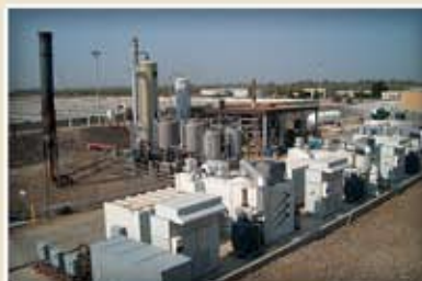
Digester Gas Fuel Cells Self Generation Incentive Program
