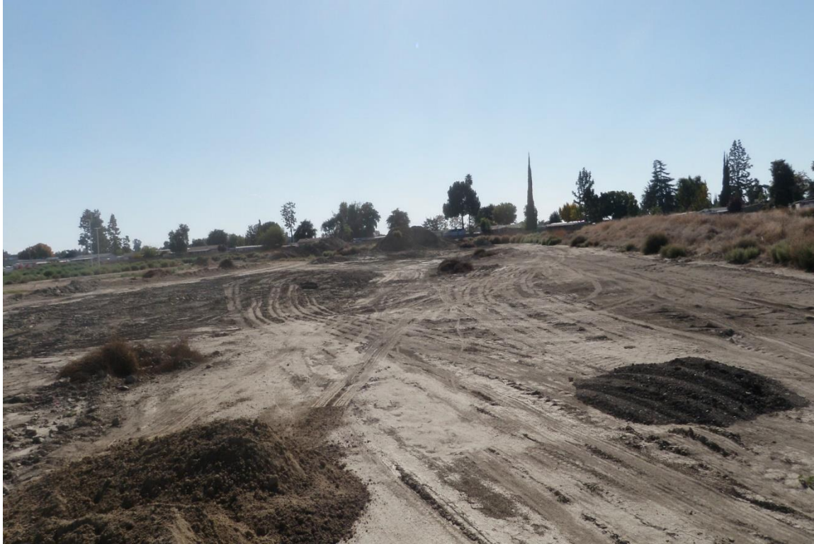
Figure 7 Overview of recent mechanical earthwork with a spoils pile at center located within the project area. South
