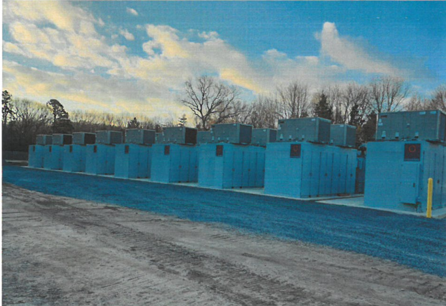
Figure 1 – Plumsted BESS (20 MW) located in New Jersey showing cabinet enclosures on concrete pads surrounded by gravel drive
