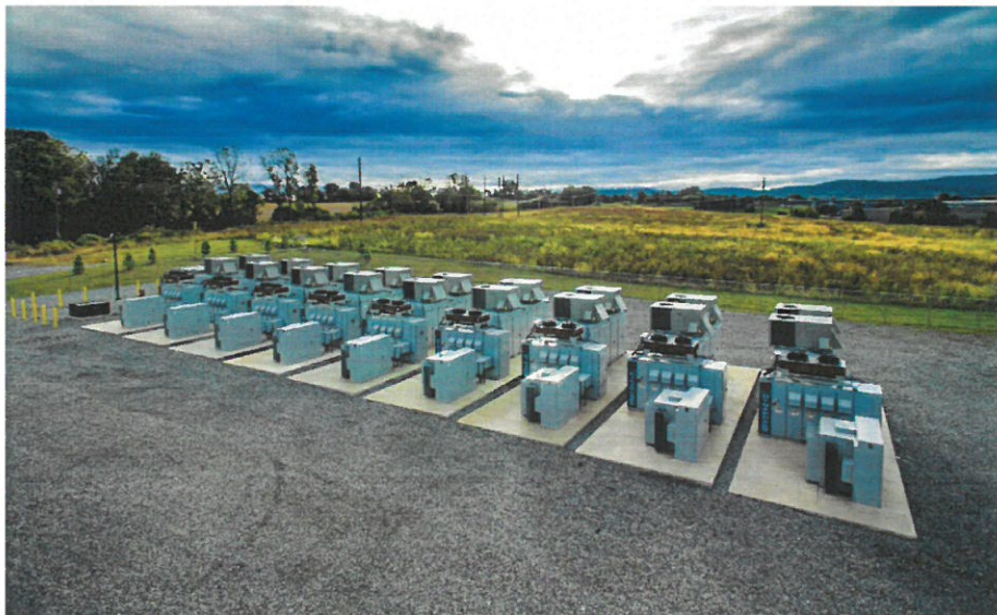
Figure 2 – Stryker BESS (20 MW) located in New Jersey showing enclosures on concrete pads surrounded by gravel apron
