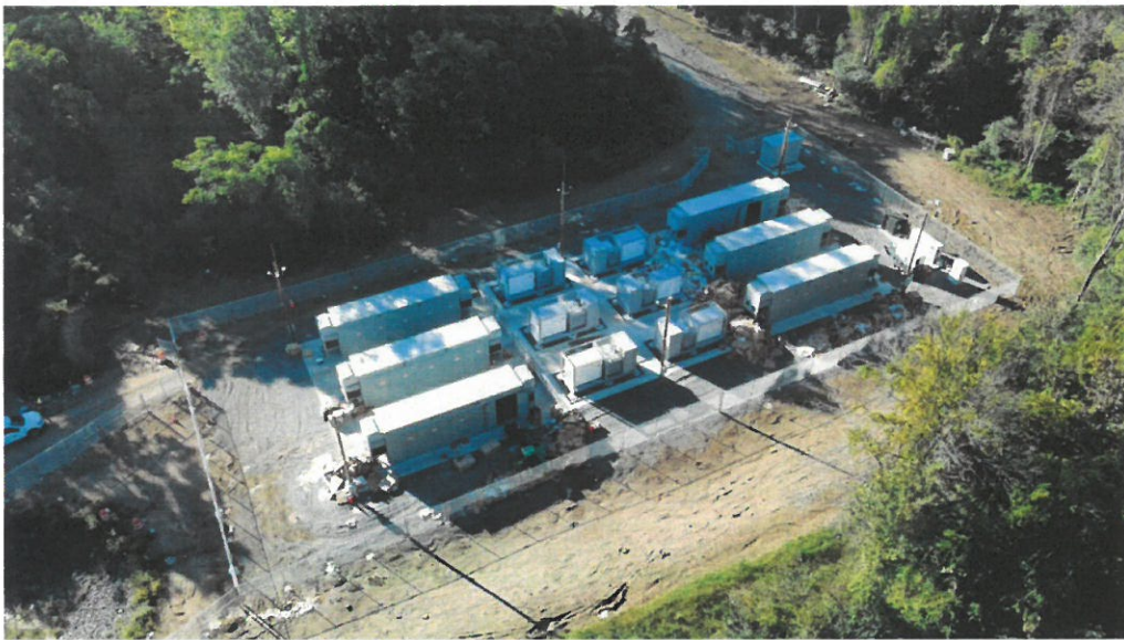
Figure 3 – Andover BESS (20 MW) in construction showing enclosures, foundations, gravel apron, fence and lighting/lightning arrester poles
