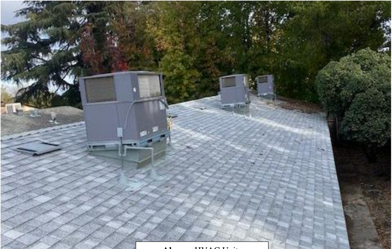
Above - HVAC Units
