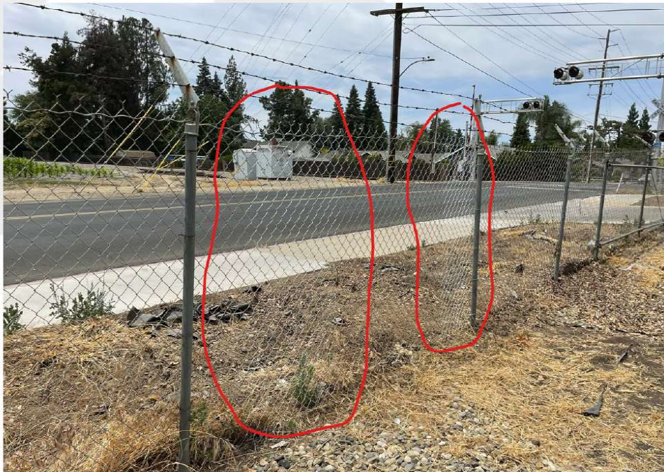
Fence repairs are a financial hardship due to ongoing criminal breach into the property.
