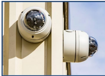
Facility Security Cameras
