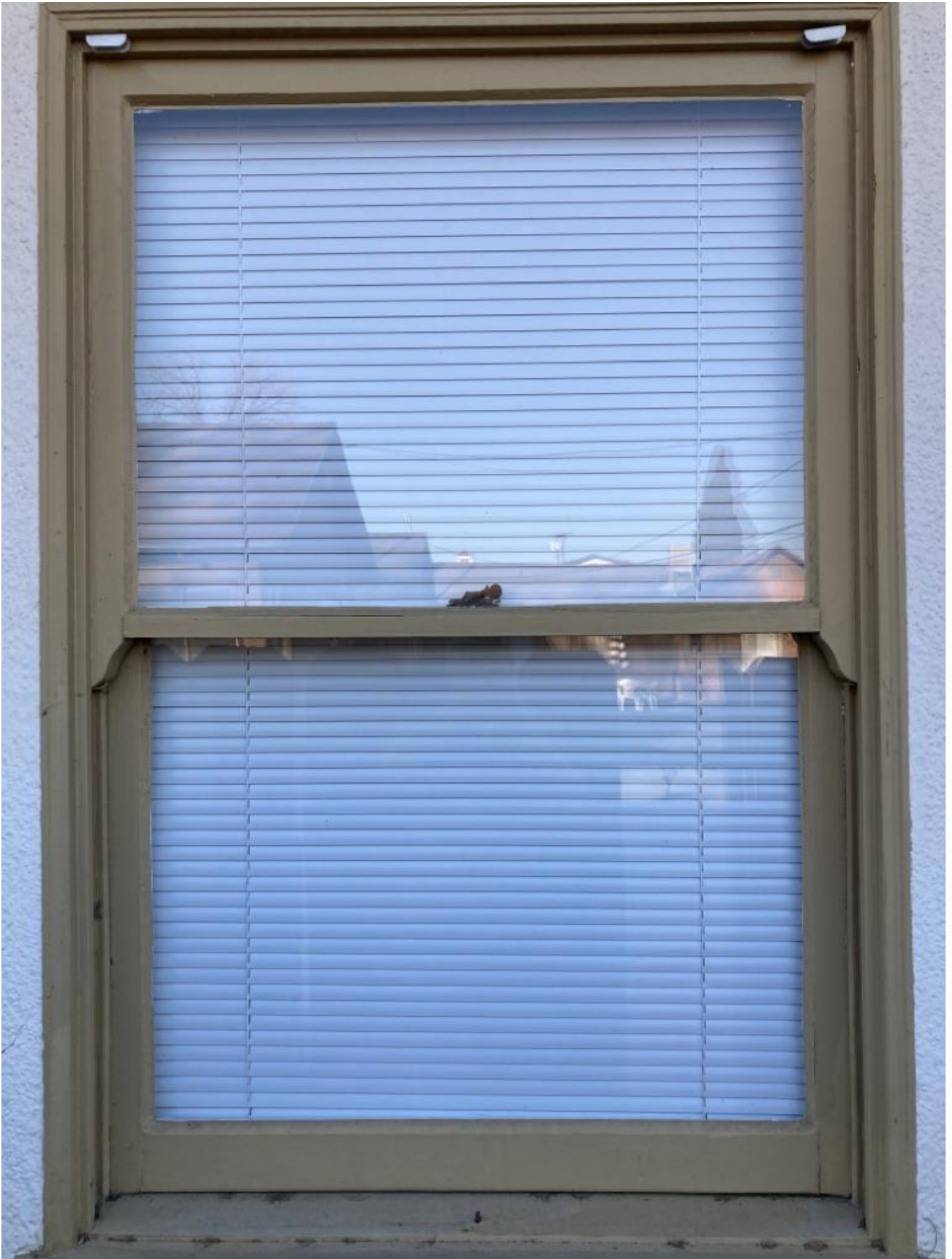
HPAC Item No. 2022-05 – Exterior Alterations
